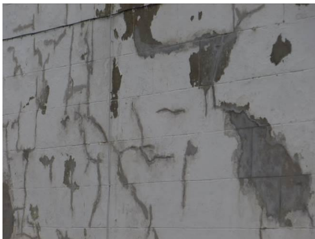
Cracked render to gable of Bullin Cottages
