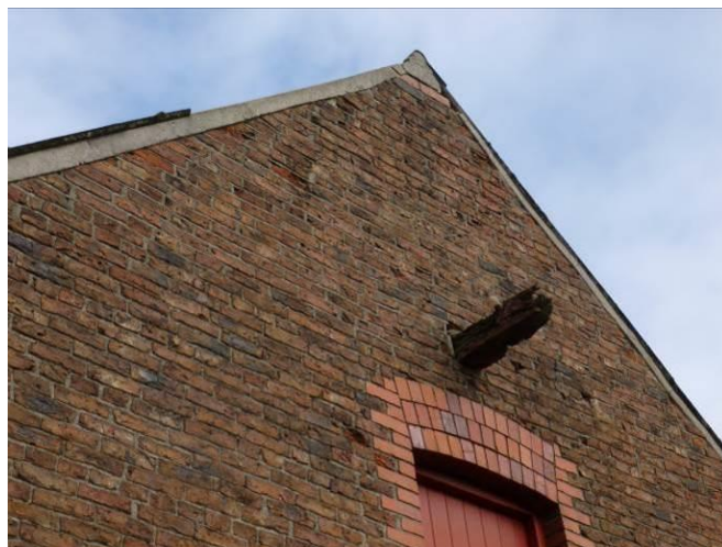
Lifting Beam to Ash Farm barn, missing roof sheet above
